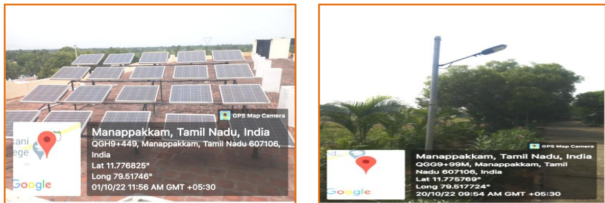
Figure 9 - Solar Panel and Street Lights
